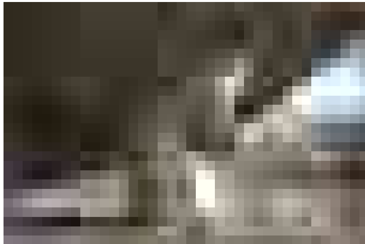
Figure D-3.2-1 Earthquake Damage (Source: FEMA)
